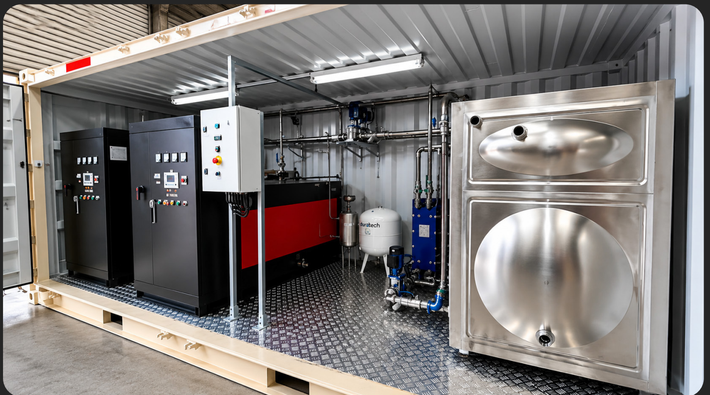
Container 2 x 180kW OBYPHASE W Heidelberg
