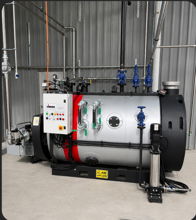
500KW OBYONE800 Steam Boiler M&KH Trading, NSW
