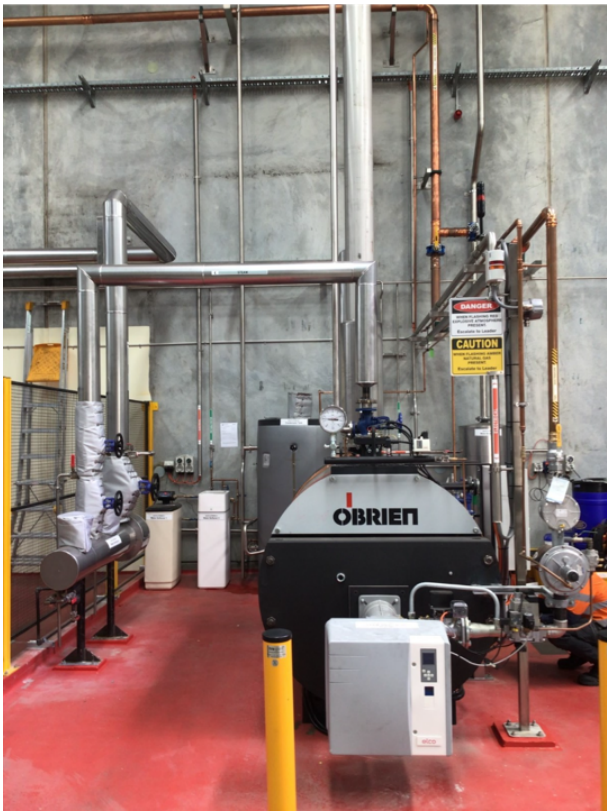
Boiler and ancillary equipment set up
