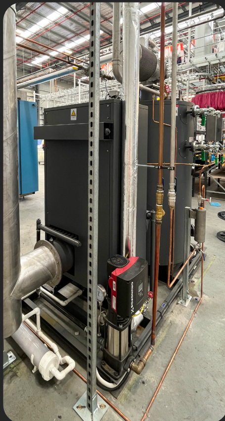
4 x 500 KW Obyvert Steam Boiler at Ensign, Truganina VIC
