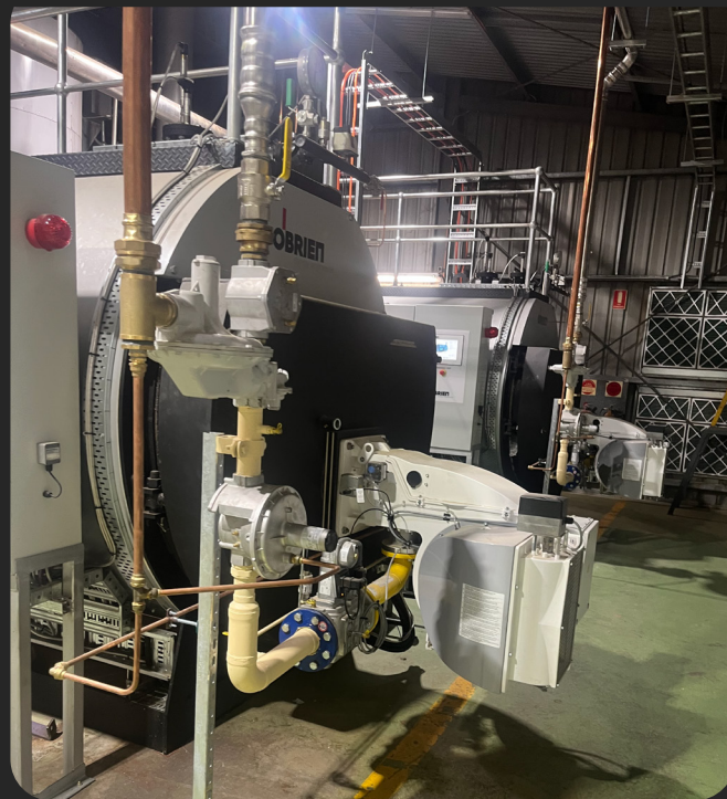
2xOBYONE S 3500 Steam Boiler JBS, 2 Regulator Rd, Yanco NSW 2703
