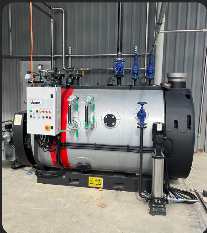
500KW OBYONE800 Steam Boiler M&KH Trading, NSW
