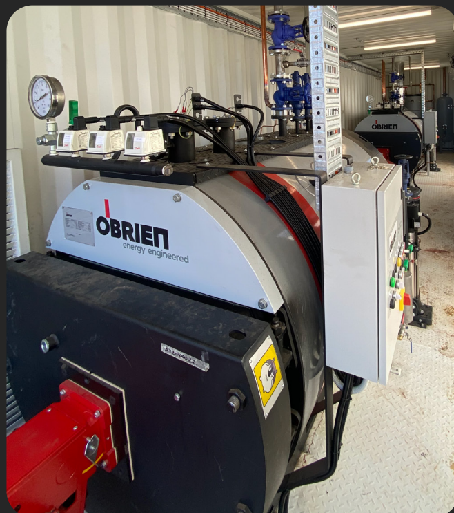
4000kW OBYONE3P-6000 Steam Boiler, Westex Investment (Western Meat Exporter), 60 Warrego Hwy, Charleville QLD
