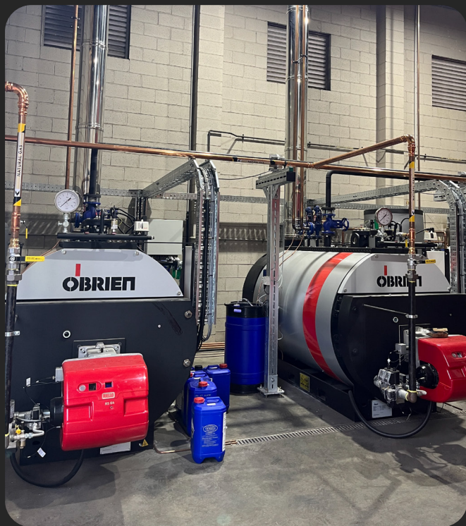
2x500kW OBYONE Steam Boiler Cleanaway, 126 Barry Road, CAMPBELLFIELD VIC 3061
